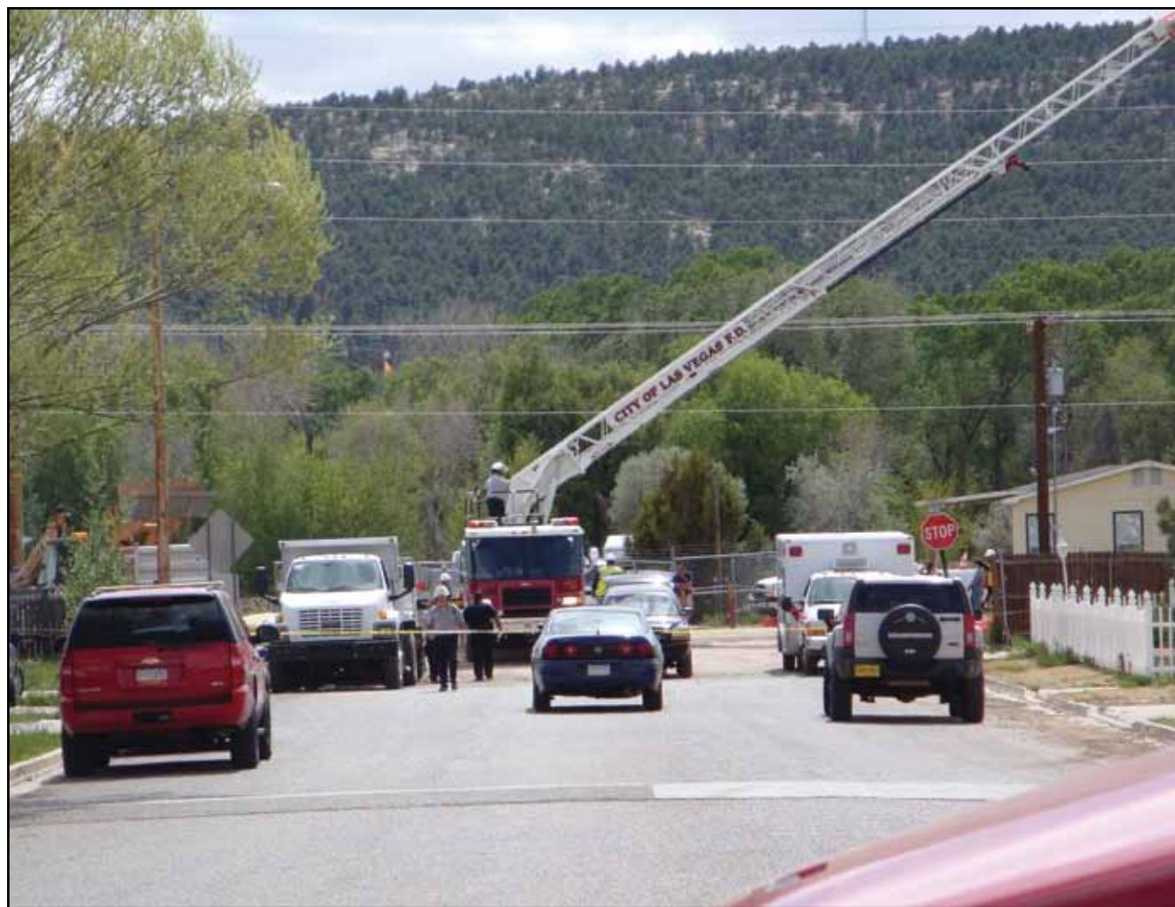
AFSCME members Gene Hern and Frank Romero were killed in Las Vegas, N.M. on May 18 when the walls of the trench they were digging collapsed on top of them.
